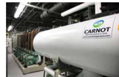
Fig. 2 Photos of the transcritical CO 2 system at Sobeys designed by Carnot Refrigeration.
