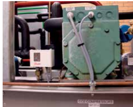
Fig. 3 CO 2 compressor in Pick'n'Pay store at Strand
