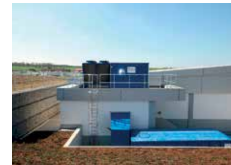
Fig. 2 Photo of Outdoor Integral Chiller Plant Installation
