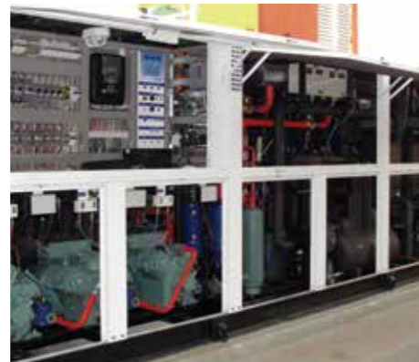
Fig. 5 The refrigeration system
