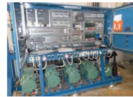
Fig. 2 The CO 2 compressor rack
